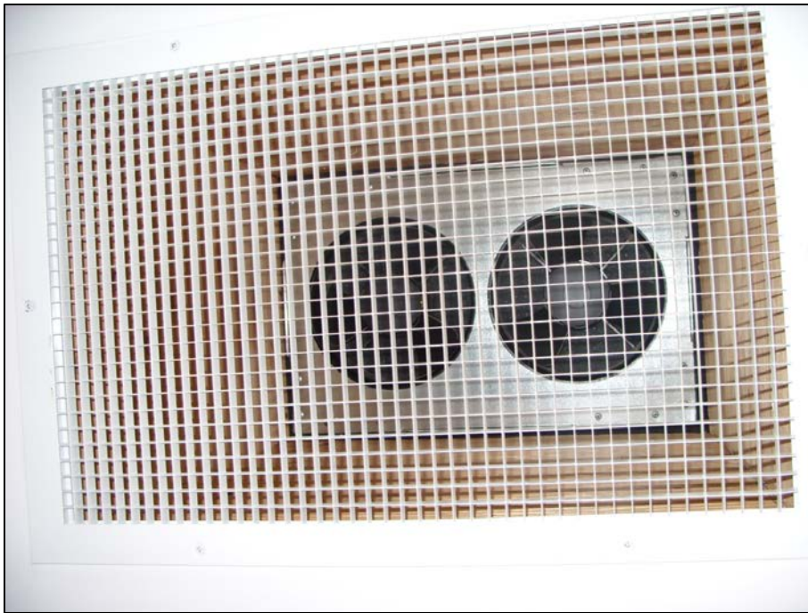
Figure 23 Whole house fan at strawbale home in ELC.
