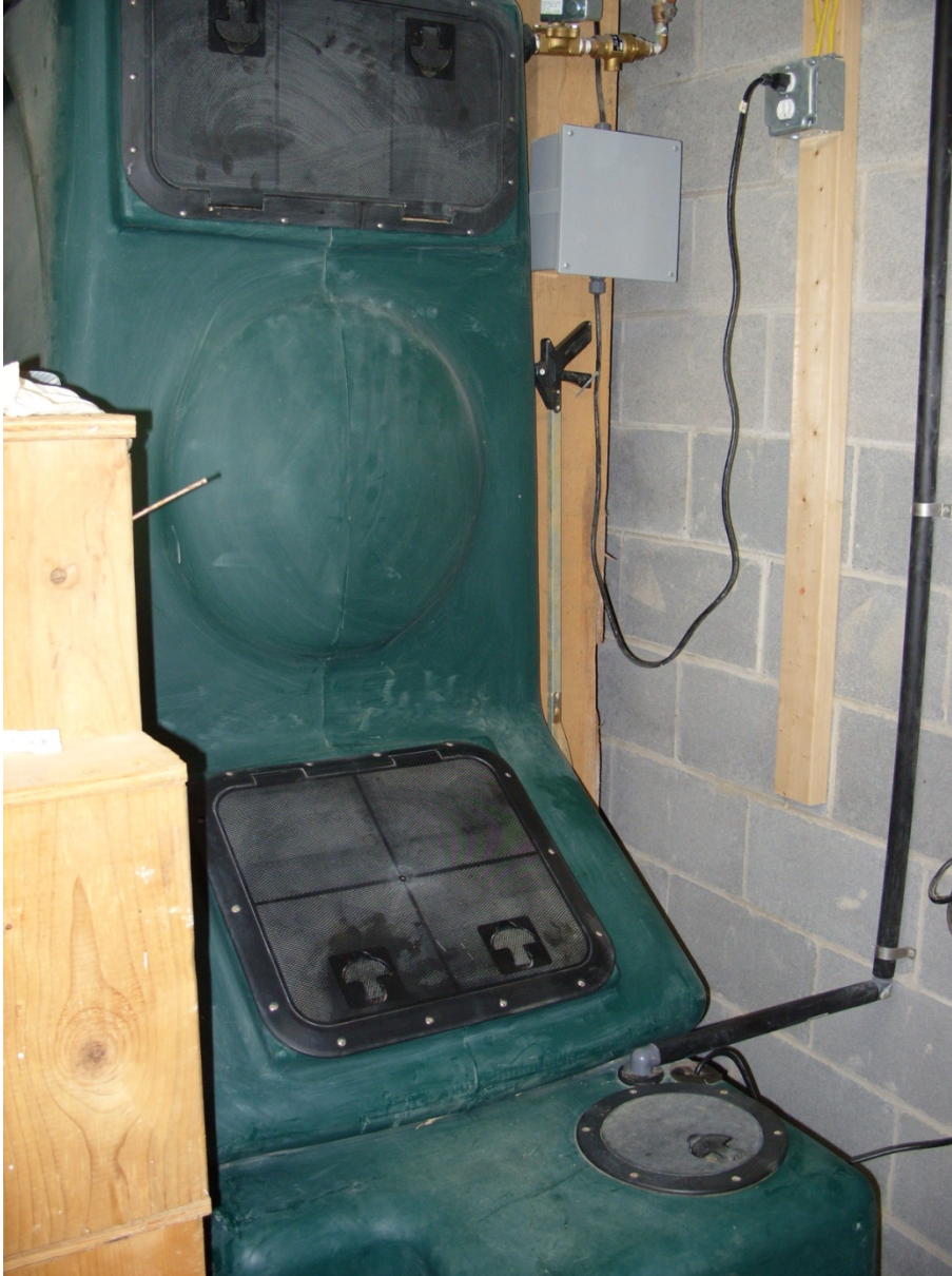
Figure 19 Composting portion of composting toilet in basement of strawbale home.
