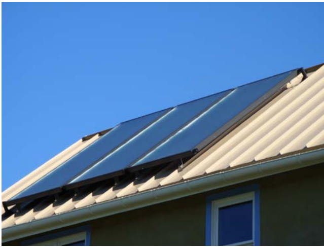
Figure 20 Solar water heater at strawbale house in ELC.
