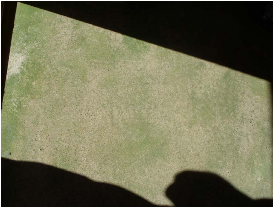
Figure 22 Concrete thermal mass floor containing hydronic radiant heating at strawbale house in ECL.
