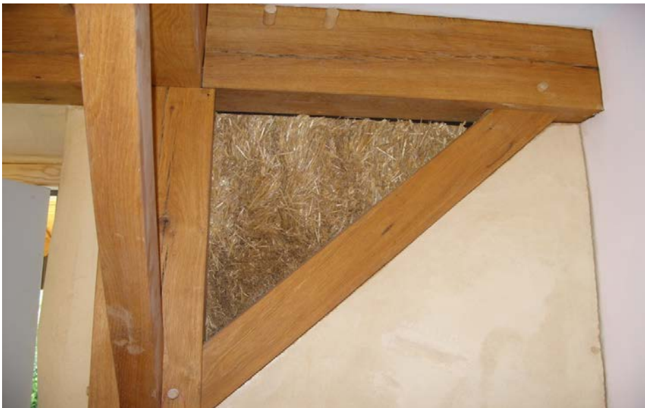
Figure 11 Wall section showing earthen plaster wall meeting timber frame supports with a "truth window" showing off the straw bale used in the wall.
